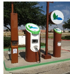
Curbside DC Fast Charging EVSE
